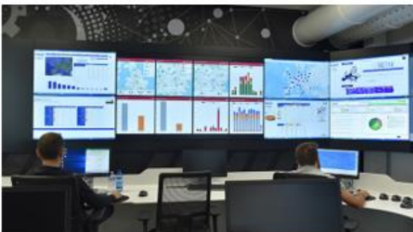
Figure 5 – 6_ CNH Industrial Control Room
